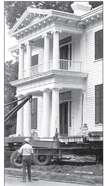
Even the two story portico of the Lewis-Smith House remained attached during its relocation.
