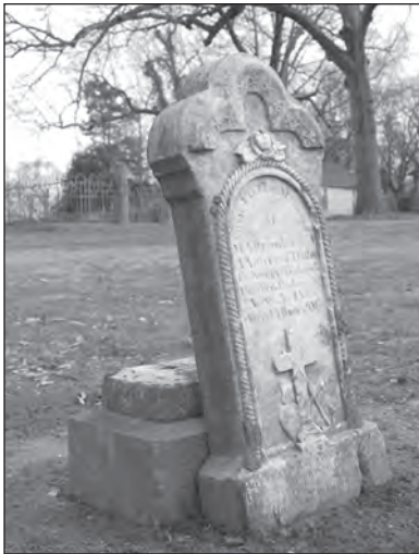
This gravestone at O'Rourke Cemetery is detached from its base. Reinstalling it could cause more damage if not overseen by an experienced stone conservator.
