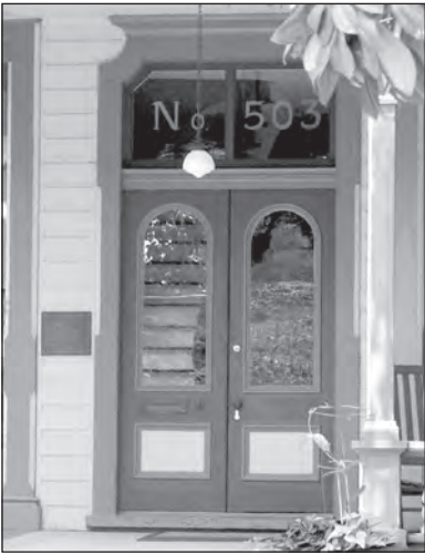
Small identification signs and historic plaques, like the one to the left of the doorway, should be located so that no significant building features or details are damaged or obscured. The glass transom provides an excellent location for displaying the street address or a business name without altering or obscuring the building facade.
