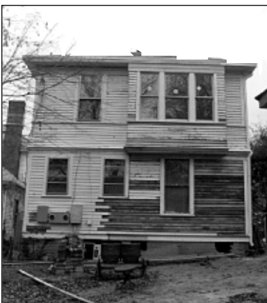
During rehabilitation, replacement siding to match the original siding was carefully incorporated on this rear facade before repainting.
