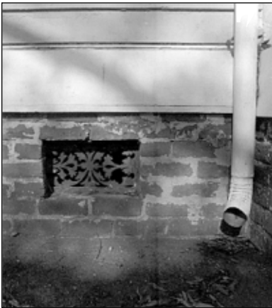
This brick foundation retains its decorative yet functional cast-iron vents. Rainwater is directed away from the foundation by the configuration of the downspout.
